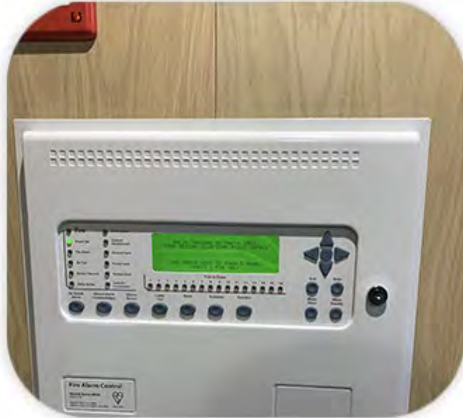
A fire alarm control panel being used as the main control panel in a mechanical smoke control system
