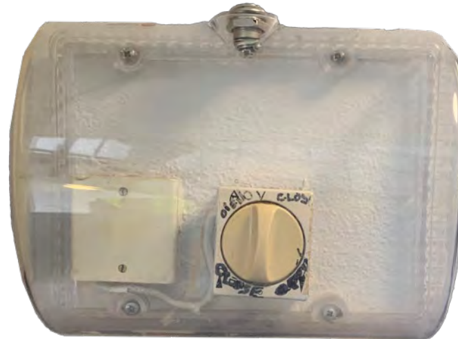
An antiquated non-compliant fireman's override switch
